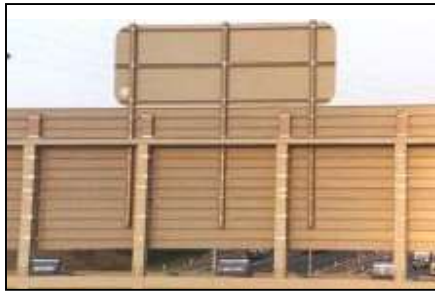
Photo: An extreme example of the use of dummy posts to extend and add a sign on a gantry
